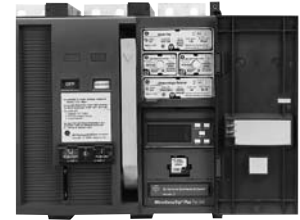
Breaker with limited access pushbutton cover assembly installed
